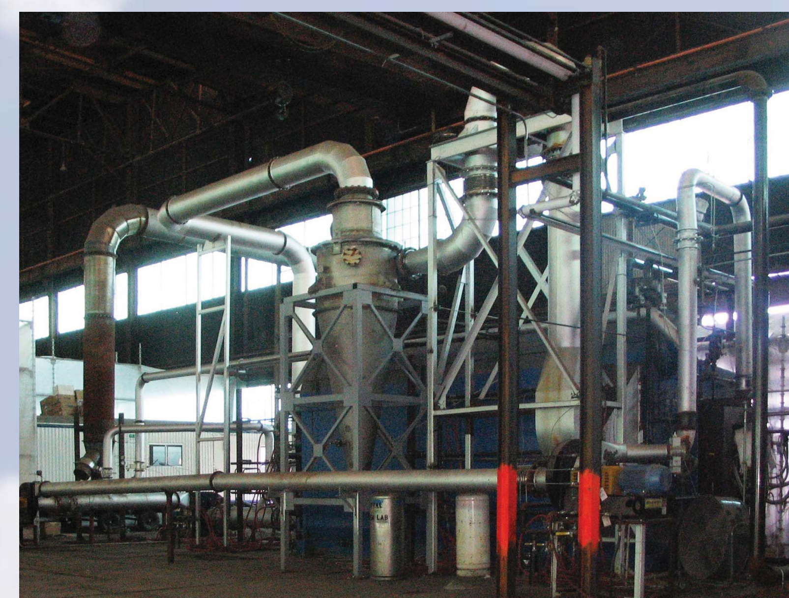
Field Demonstration of Oxy-Combustion Burner Test and IPR ™
