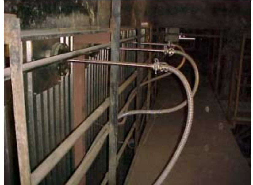
Mercury Sorbent Injection Ports at Southern Company's Gaston Station
