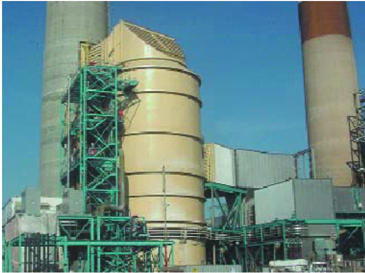
Wet FGD Scrubber
