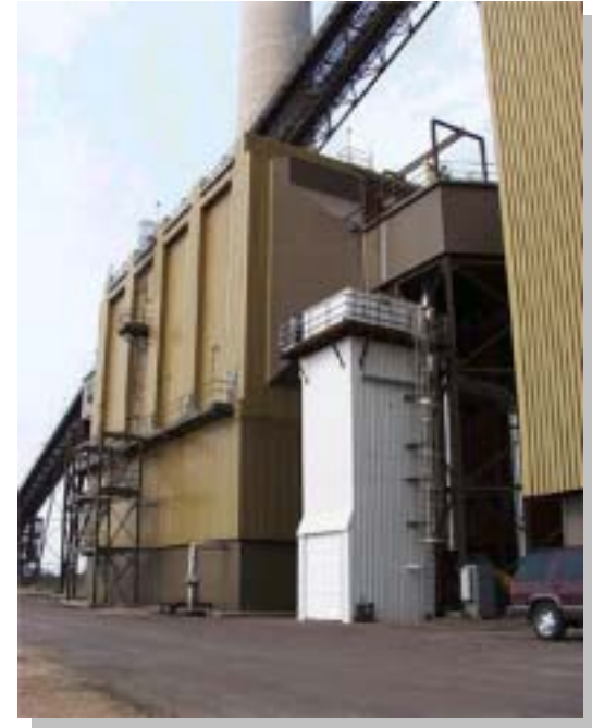
AHPC Slipstream Test Unit at Big Stone Power Plant
