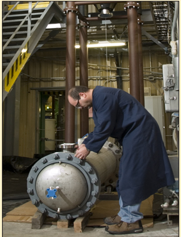
Equipment installation is under way at the SRNL Pilot Test Facility where Fractional Crystallization will be tested in 2008.
