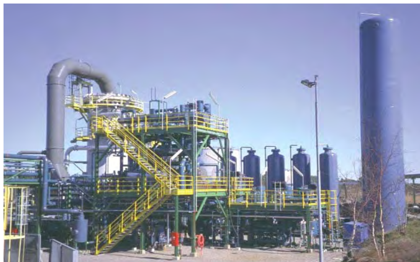
Figure 3B-1. Steam-Methane Reforming Plant (Axsia Howmar plant in Sweden)
