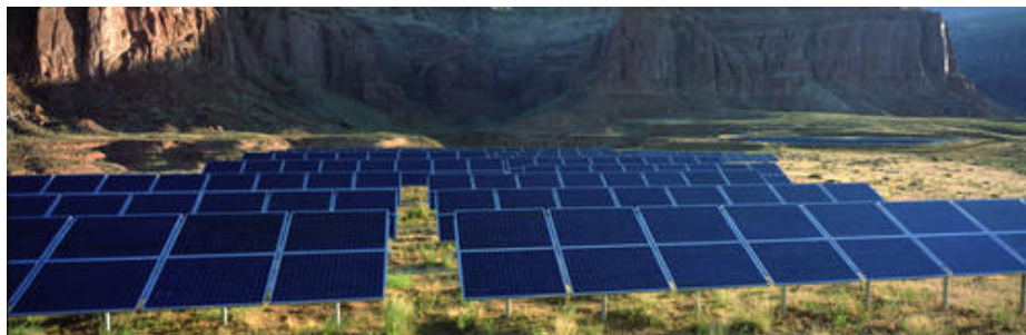
Solar Photovoltaic Power Plant
