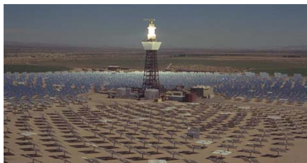
Solar Power Tower
