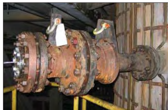
Sapphire sensors packaged into a probe (shown here) were installed and tested at Tampa Electric's Polk Power Station
