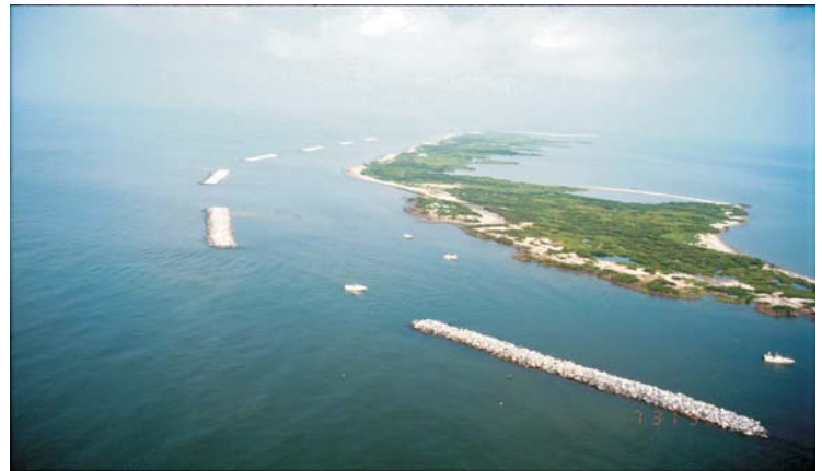
Rock breakwater construction for the prior demonstration phase of this project was completed on the east end of the island in June 1997. Taken immediately after construction was complete, this 1997 photograph shows no sand behind the breakwaters.
