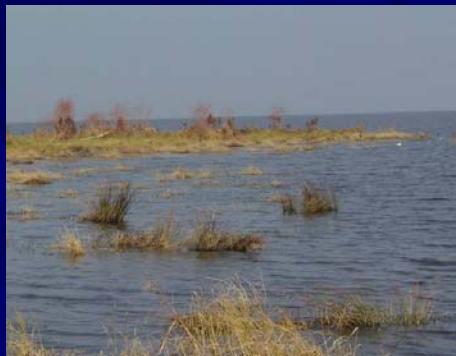
Significant shoreline erosion after Hurricane Katrina at South Shore of The Pen – protection feature not yet constructed. Note eroded marsh in foreground and deposited on remaining marsh
