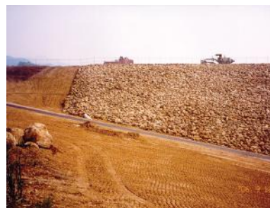
Construction to reduce the risk of damage to Lauro Dam from a major earthquake was completed in 2006
