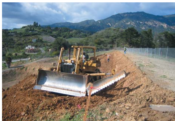
Lauro Dam modification in late 2005 near Santa Barbara, California, under the Safety of Dams Program
