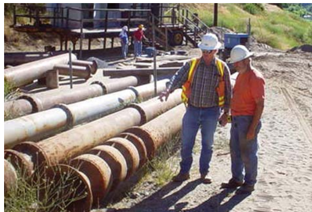
Dennis Edwards (L), construction Inspector from the Mid-Pacific Construction Office in Willows, California, shows contractor Tony Lynn of Berkeley Engineering (R) temporary water pumps to be used to provide the Placer County Water Agency with water from the American River North Fork near Auburn, California.
