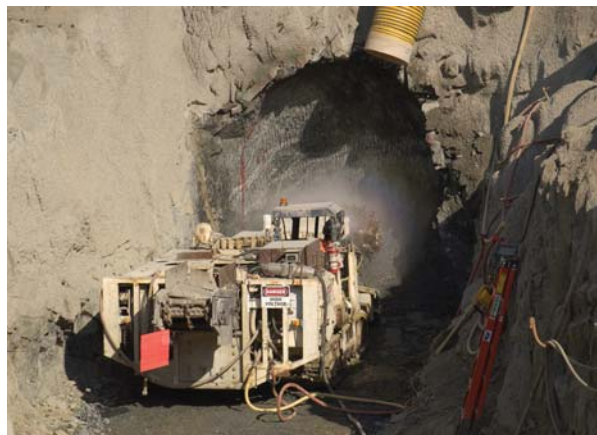
Contractors work on the tunnel leading to the pumping plant in early 2005.
