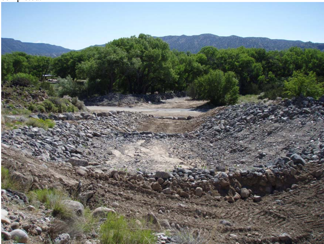
Photo 4. The arroyo downstream of the quarry area following recent repairs (June 2007).
