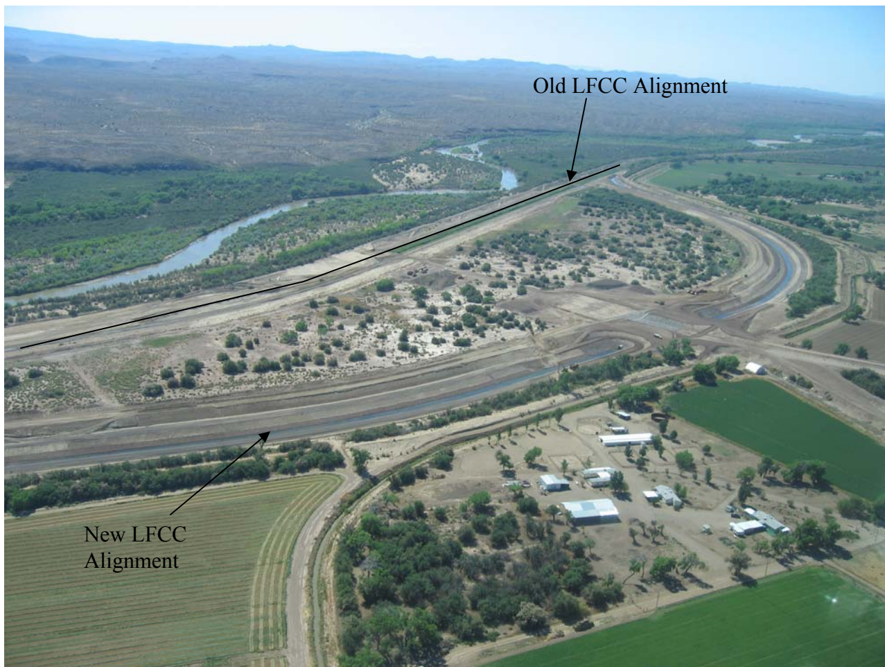
Photo 10. Looking downstream at the new LFCC in the area of River Mile 113/114 Priority Site (May 2006)
