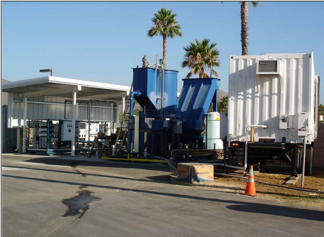
Figure 3.2 Site layout of RO skid, Zimpro softening unit, and EDR trailer.
