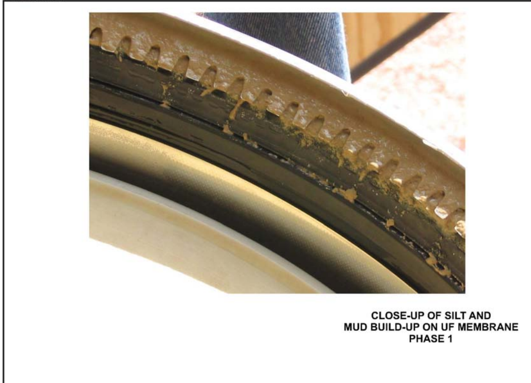
Figure 5.5 Close-Up of Silt and Mud Build-Up on UF Membrane Phase 1.
