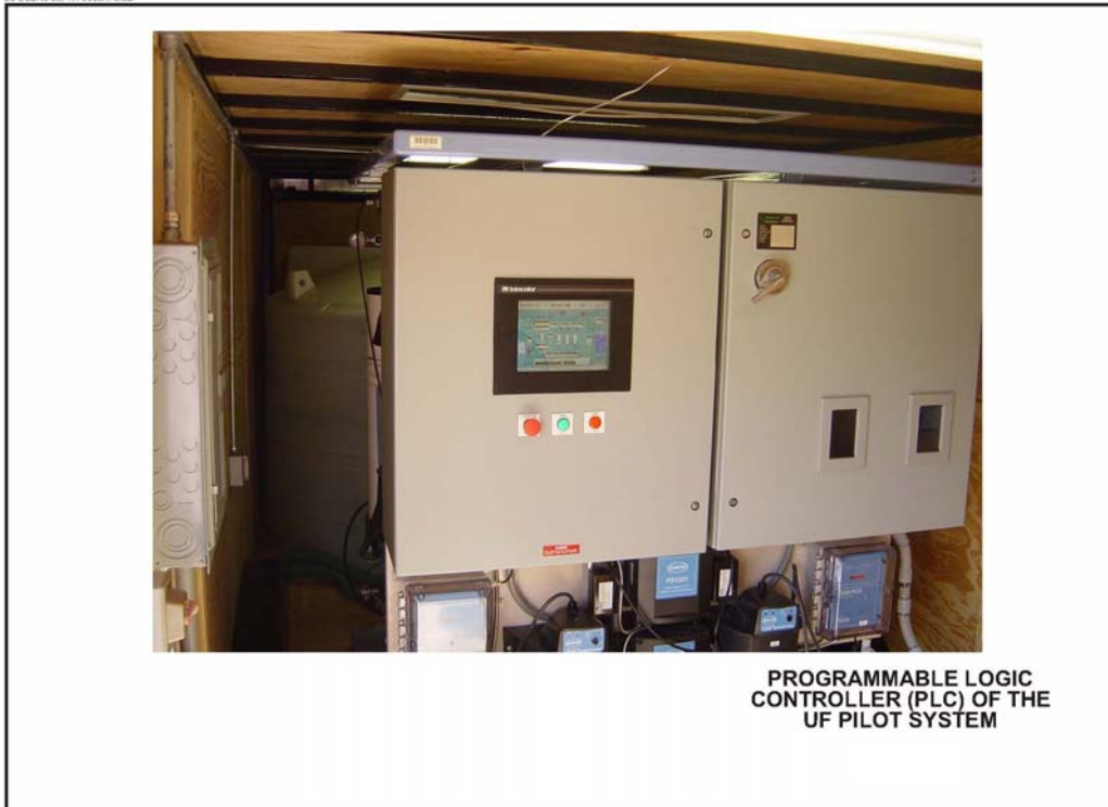
Figure 4.4 Programmable Logic Controller (PLC) of the UF Pilot System.
