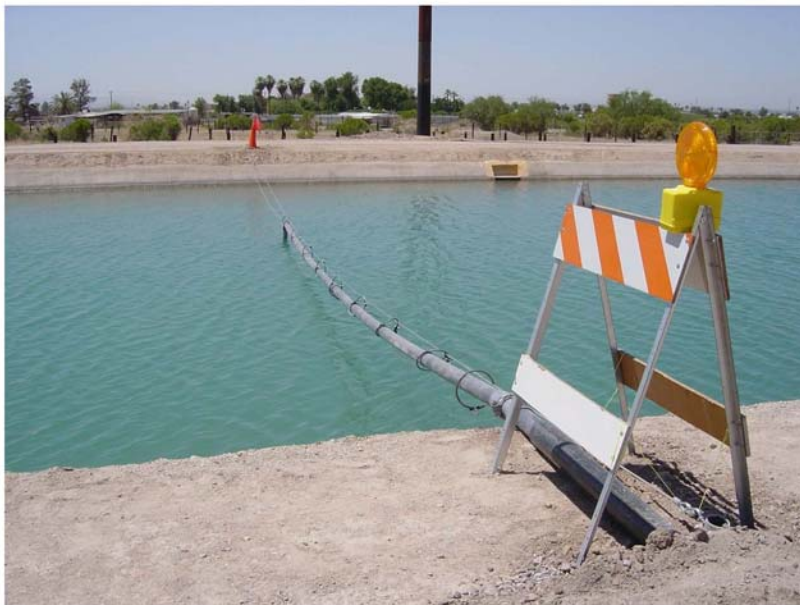
RAW WATER INTAKE PIPING
