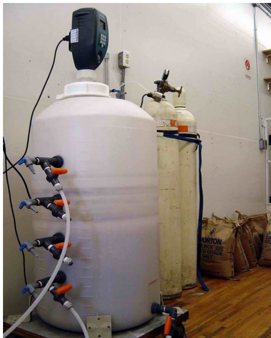
Figure 4-4. Biological brine treatment system.
