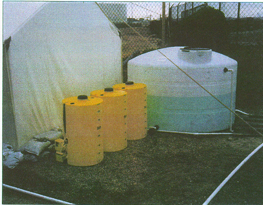
Figure 8. Chemical Injection System.
