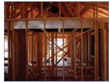
Carefully designed duct runs, placed in interior spaces, save energy and help maintain comfort.
