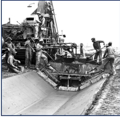
View of freshly laid plastic soil-cement canal lining in West 11.5 Lateral, May 5, 1947. The paver and mixer traveled at a rate of five feet per minute while soil-cement material was distributed into the hopper by hand (National Archives and Records Administration 1947a). This and other low-cost liner applications were used to minimize water loss in high seepage areas of the canal and lateral system.
