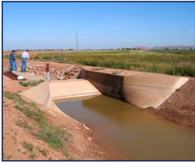
View of a recently installed measurement structure in the West Canal, October 13, 2004. This broad-crested weir allows more accurate measurement of flow from the Main Canal into the West Canal. Photograph courtesy of Bureau of Reclamation, Austin, Texas.
