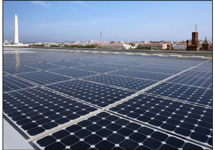
A view of a portion of the 891 individual solar panels now generating electricity on the Forrestal roof
