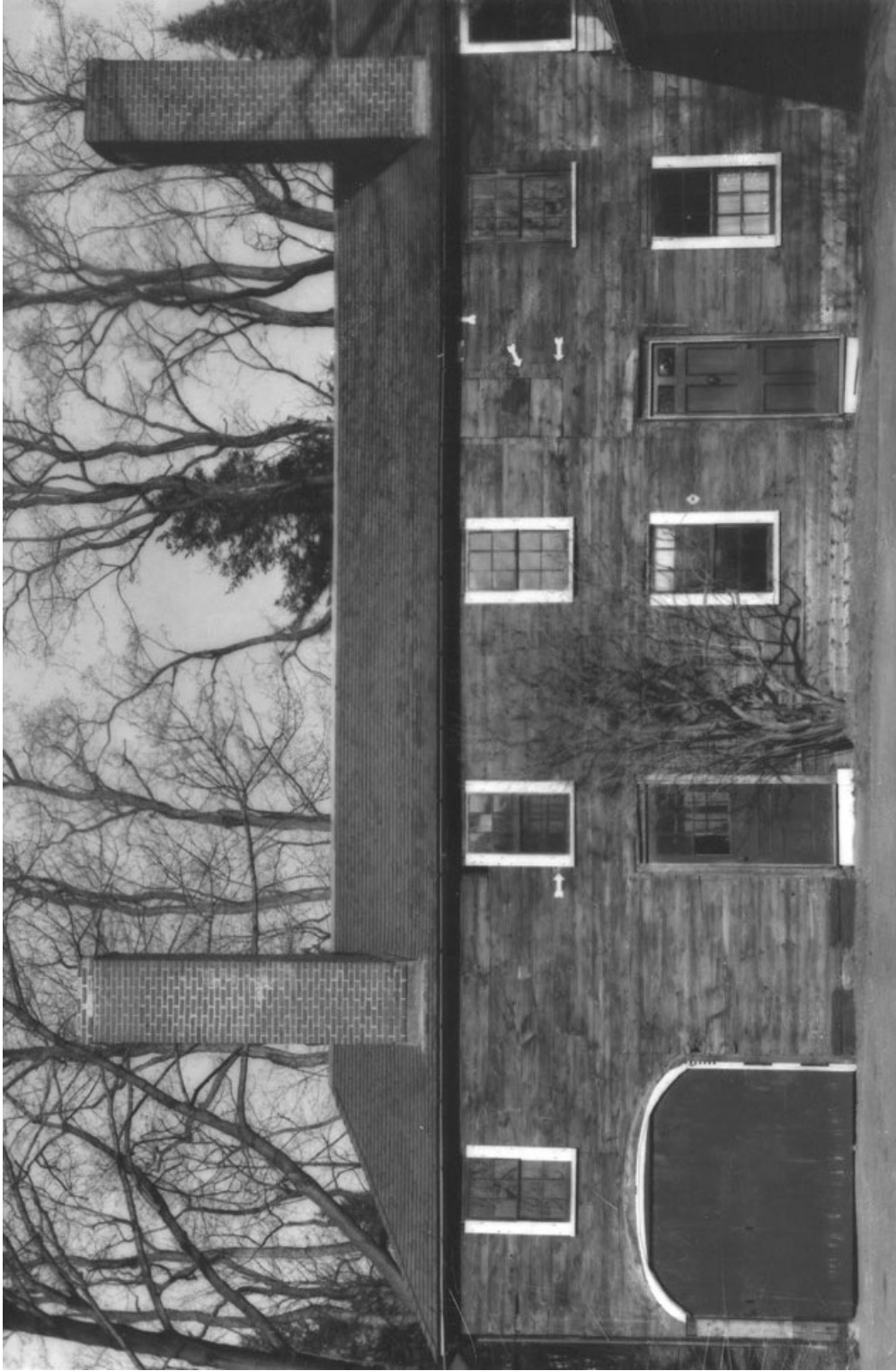
Figure 18. Elisha Jones Shed: West elevation, with arrows indicating evidence of original window openings. The left window (W224) was reused by John Keyes, and the right one was boarded over in 1865.
