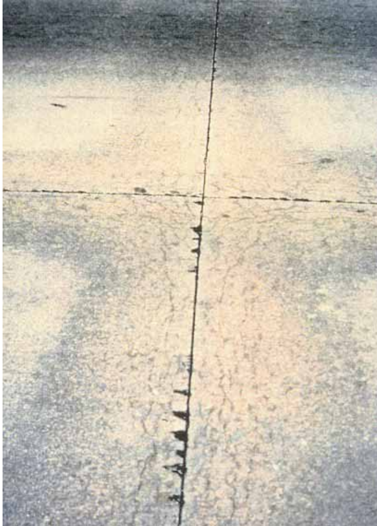
Figure 221. D-cracking of a pavement caused by destruction of the aggregate by cycles of freezing and thawing (cracking parallel to the joint and wrapping around at the juncture of joints defines D-cracking).
