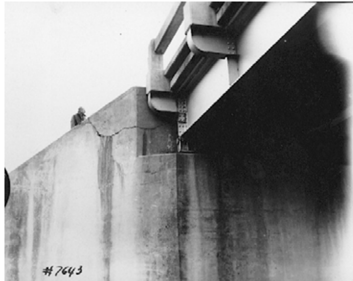
Figure 98. Upper portion of backwall sheared by expansion of bridge deck.
