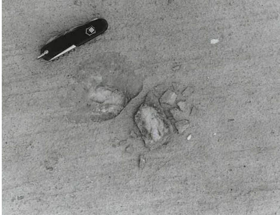
Figure 222. Pavement surface with a flaw caused by freezing and thawing of water trapped in aggregate particle.
