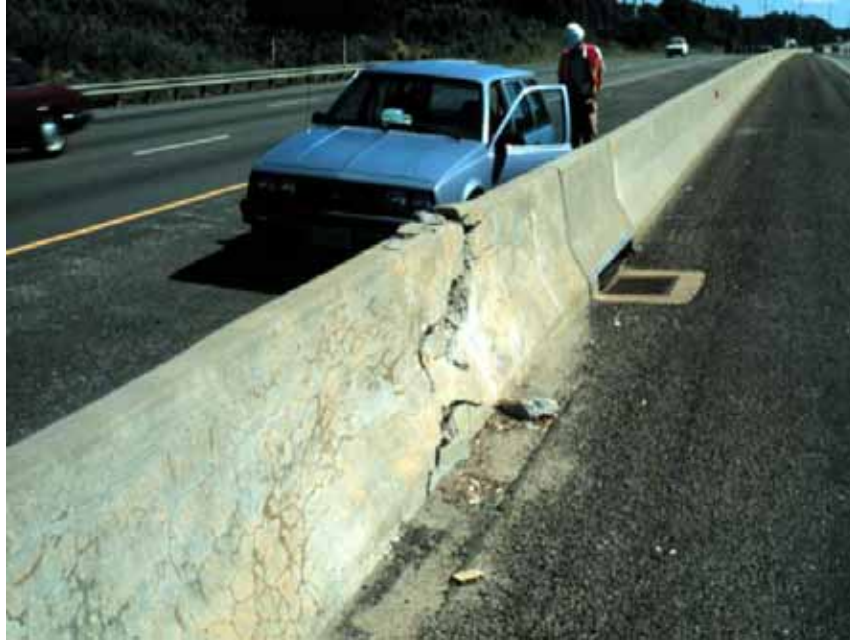
Expansion caused by ASR of quartzose coarse aggregate.
