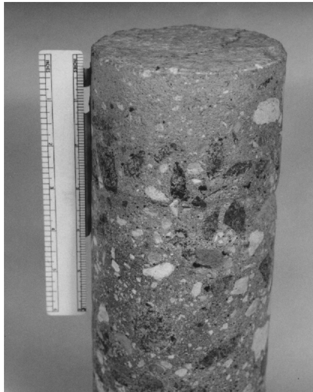
Figure 76. Overwatered concrete: Rain and snow occurring after the concrete was placed caused overwatering near the surface (top). (The aggregate sunk out of the overwatered zone.)
