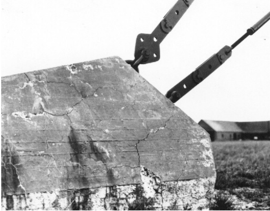
Figure 96. Destructive ASR in anchor block.
