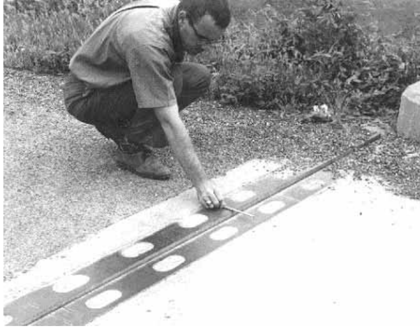
Figure 100. Closing of joint caused by bridge deck expansion as a result of ACR.
