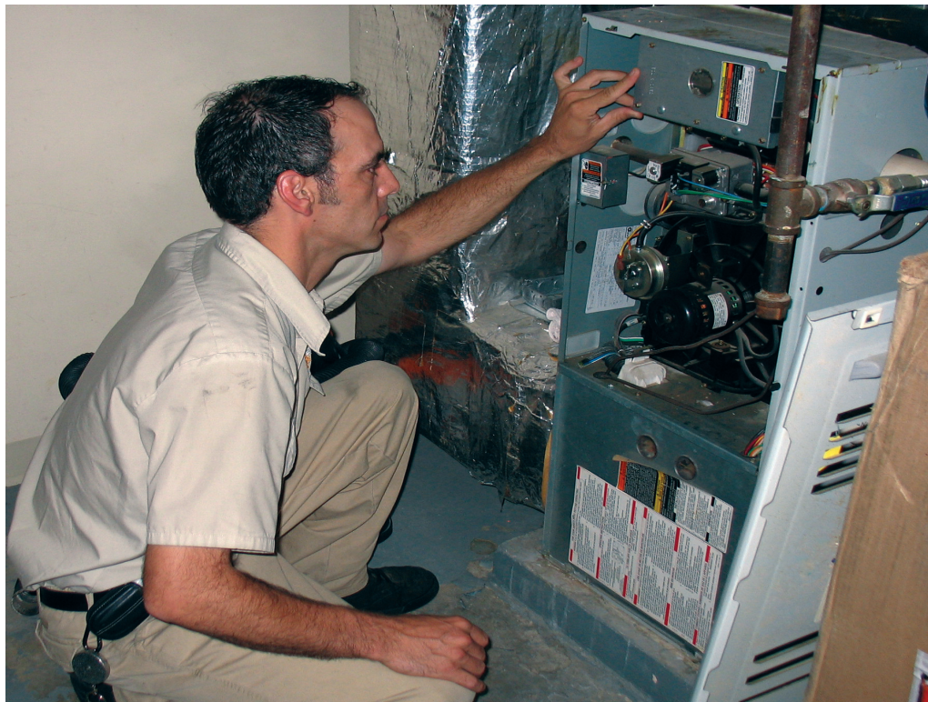
Dan Jones, Maintenance Technician Extended Stay Hotel, Greensboro
