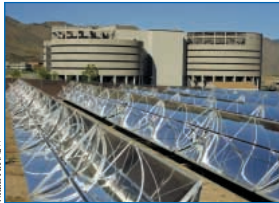
Installed in 1997, the hot water system at the Jefferson County Jail in Golden, Colorado, uses trough collectors and produces 50% of the hot water used annually in the facility.
