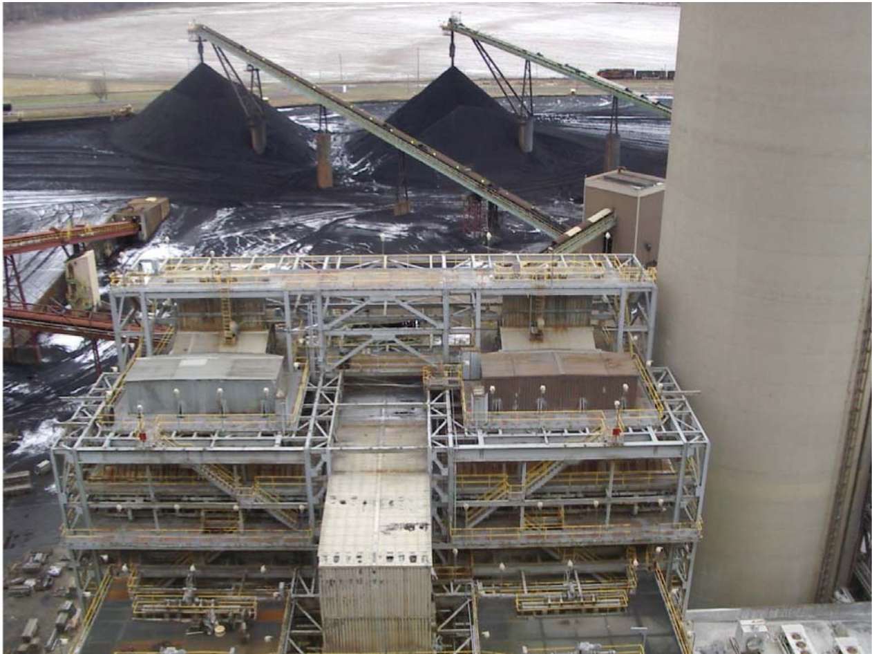
Figure 3-14: Conesville Unit #5 Existing Flue Gas Desulfurization System Scrubbers and Stack
