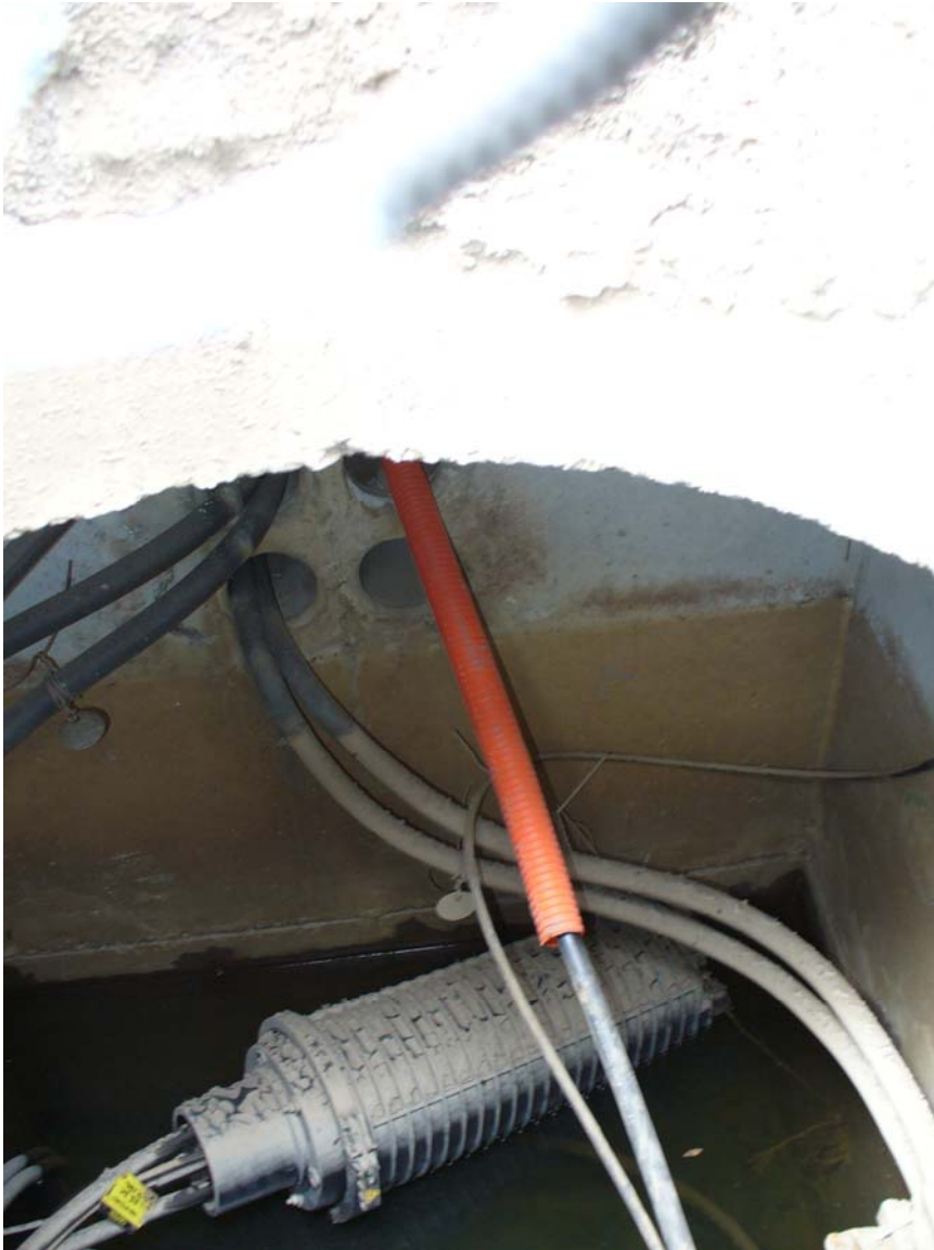
Figure 7: City Fiber Optic Cable In MTA MUNI Conduit and Manhole
