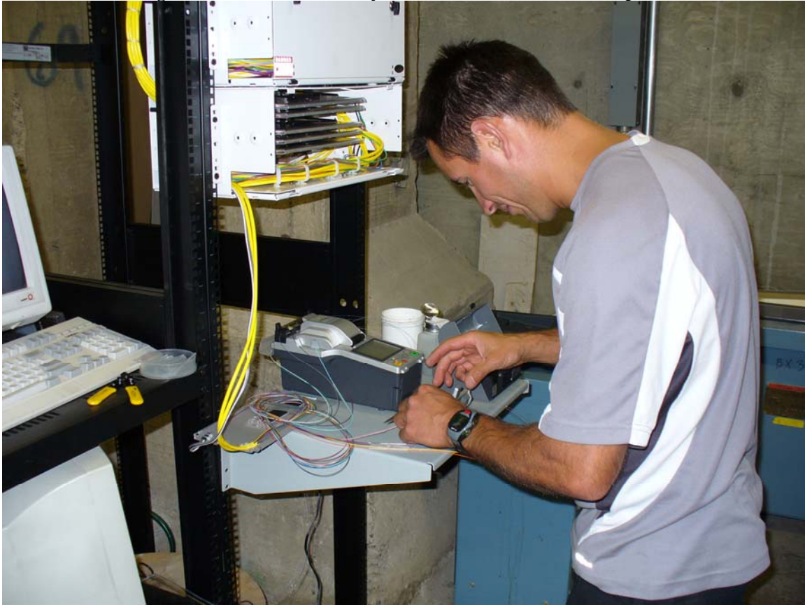
Figure 11: DTIS Public Safety Outside Wire Division Fiber Splicer
