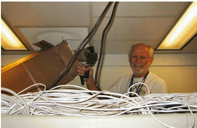
Graham Stork, IT Computer Systems Manager, turns packaging tape and a cardboard box into a "state-of-the-art" temporary cold air duct to route cool air to overheating switches.
