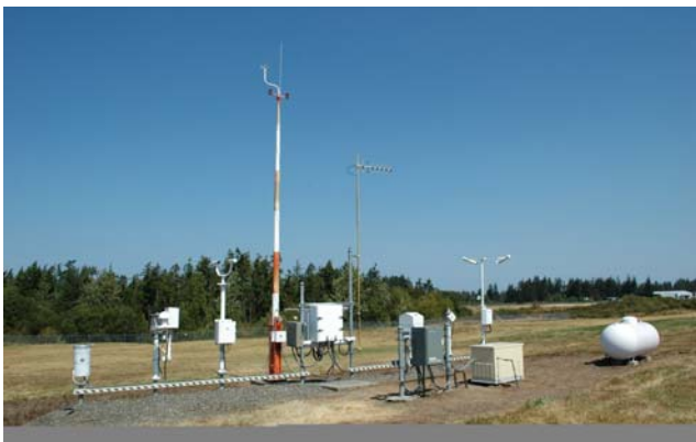
Port Angeles, WA ASOS site with new backup generator
