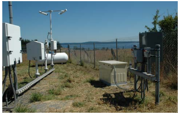
Friday Harbor, WA ASOS site with new generator.
