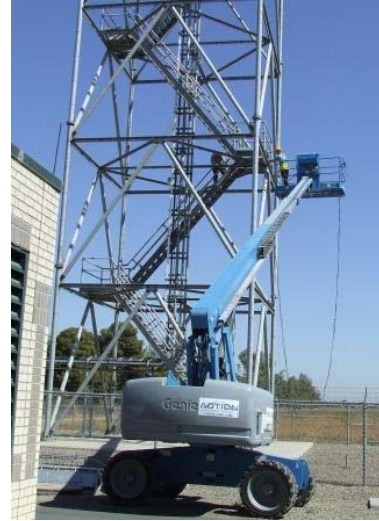
Pictured are ET's Tim Johnson (on the tower) and Marc Ganey (on the lift) installing the new equipment. Not pictured is FET Jim MacLellan, who was also involved in the project.
