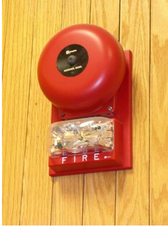
Figure: Audible and visual fire alarm
