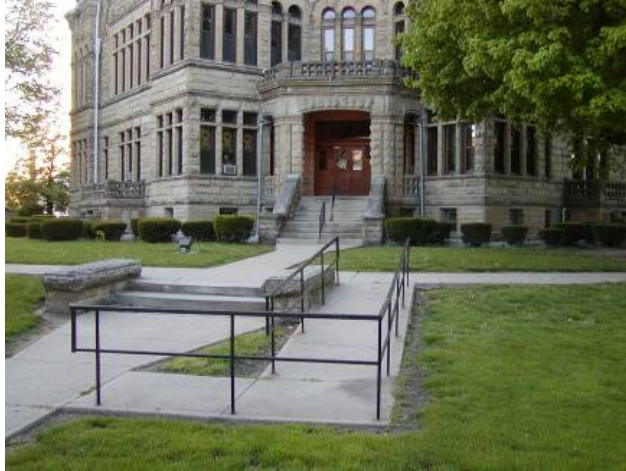
Figure: This exterior ramp is located along the same general path of travel as provided for the general public. However, while the ramp does provide handrails, it does not have edge protection.
