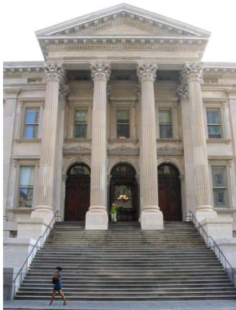
Figure: Plinth with stairs creating access problems
