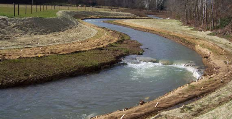
Recently restored section of Brushy Creek. Note the structure which helps hold grade allowing for riffle-pool formation, and the new floodplain area (matting and staking) providing overflow.
