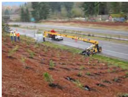
WSDOT is restoring more than 63 acres of roadside affected by the SR 18 widening project
