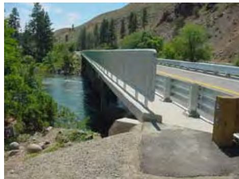
AFTER: The replacement bridge rail meets current safety standards, and greatly reduces the possibility of vehicle penetration.
