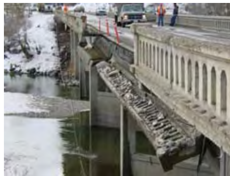
BEFORE: Nonstandard bridge rail on SR153 near Carlton, Washington. This illustrates the safety risk posed by nonstandard bridge rail
