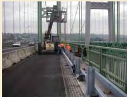
Crews install the new guardrail on the south side of the 1950 bridge.
