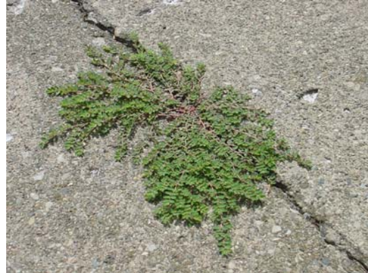
Fig 2 Spurge growing in a crack in the sidewalk.
