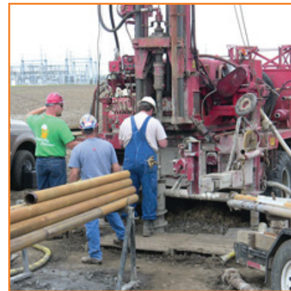
ISGS drilling and well installation at the ADM site for the monitoring, mitigation, and verification portion of the deep saline reservoir pilot program.
