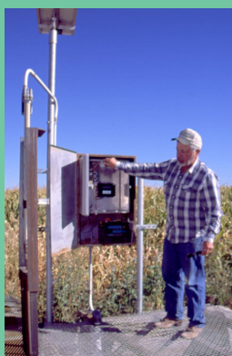
George Davis fashioned an automatic solar-powered irrigation water diversion gate using off-the-shelf components.
