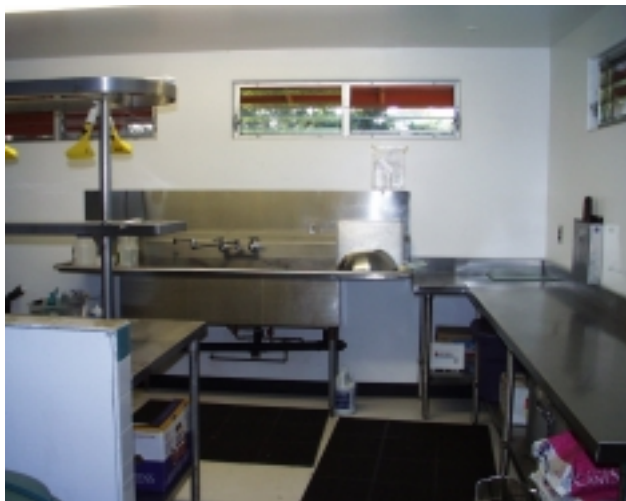
Food-preparation sink with stainless-steel countertop.
