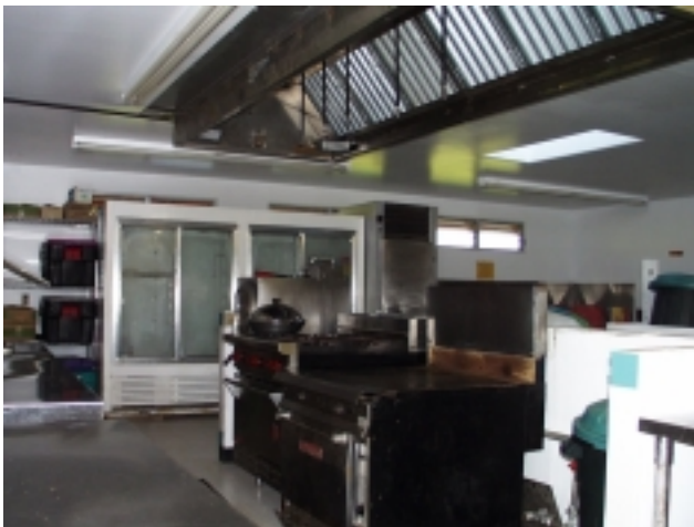
An exhaust hood vents fumes from cooking surfaces.
