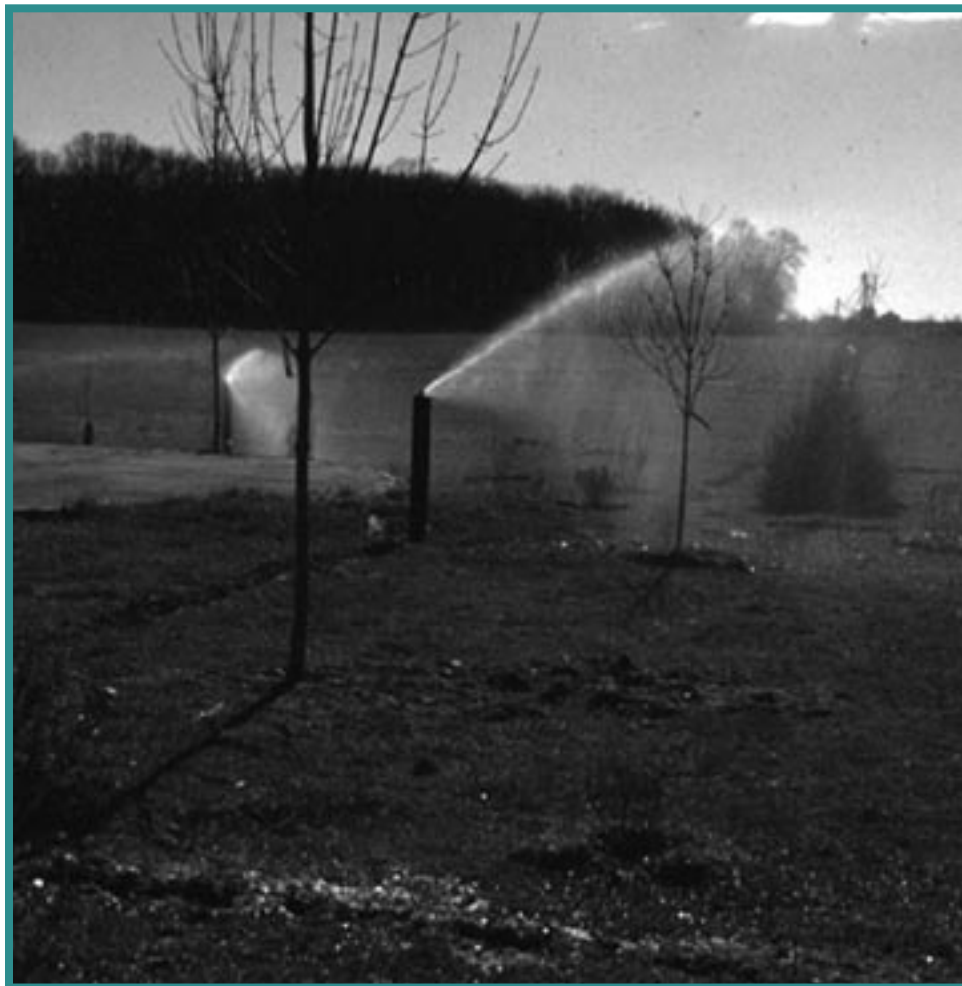
Onsite wastewater irrigation system serving a 3-bedroom home at the OSU Molly Caren Agricultural Center near London, Ohio.
