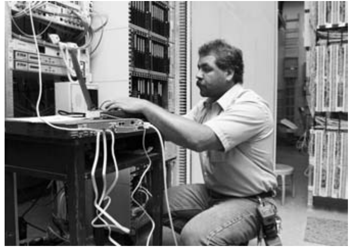
Telecommunications equipment installers make adjustments in central offices.
