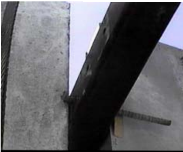
Figure 1. Finger rack with inadequate rebar pin holding panels. Also the pin is not properly placed
