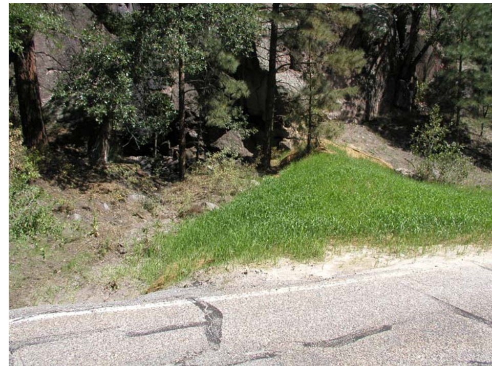
Figure 3.1-2 Earthen berm that routes stormwater under paved road through 18-in. culvert and away from LA-SMA-2 drainage
