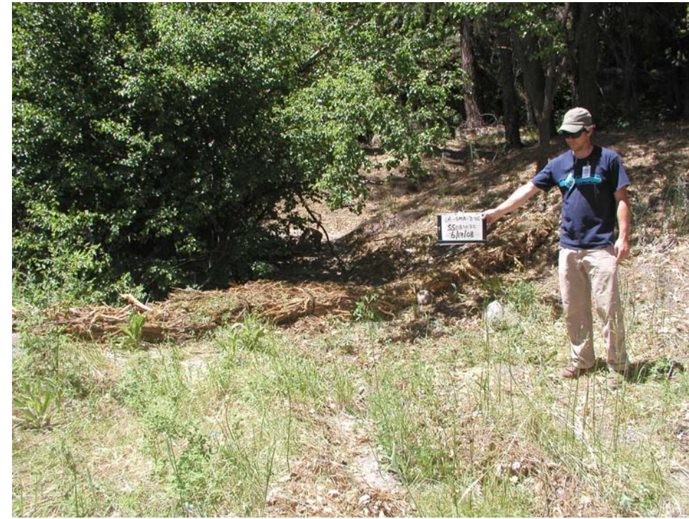
Figure 3.1-1 Example of juniper bales placed below LA-SMA-2 FFCA sampler and above the LA-SMA-2.15 sampler
