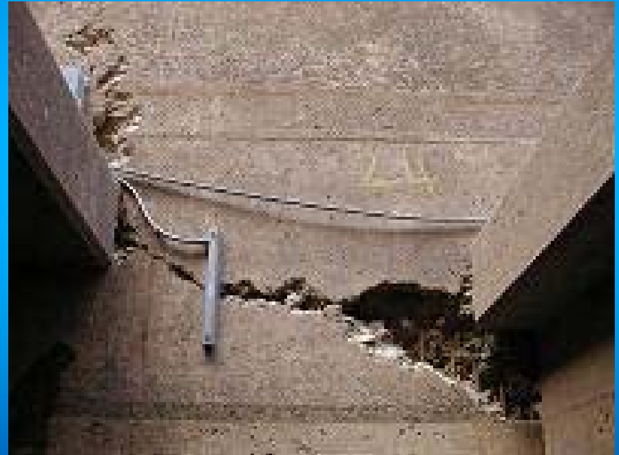
Horizontal cracking on monolith bases
