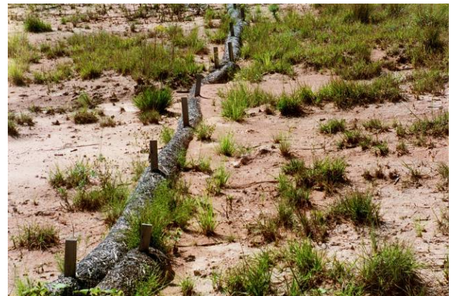
Giant sacaton erosion control planting at the Hobbs, New Mexico landfill site as of September 2007. Waddles were previously installed to help against water erosion.
