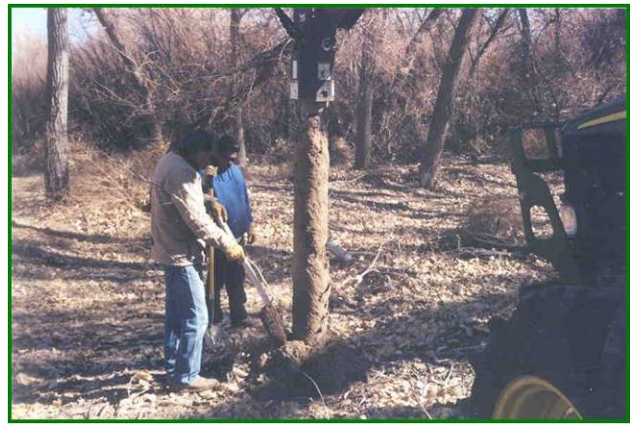
Placing the rootball at a 5-foot depth in order to come in contact with the capillary water.
