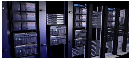
Photo: A state-of-the-art data center with rack mounted servers (image courtesy of Python).
