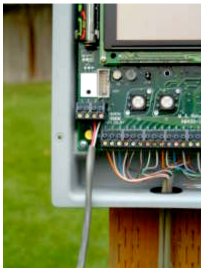
Downloading cable connected. (M. K. Hansen Company)
