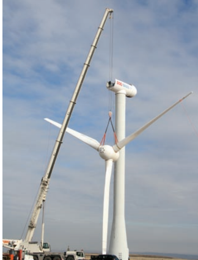
NWTC team member, Garth Johnson, works in the rotor's hub after it is installed on the turbine.
