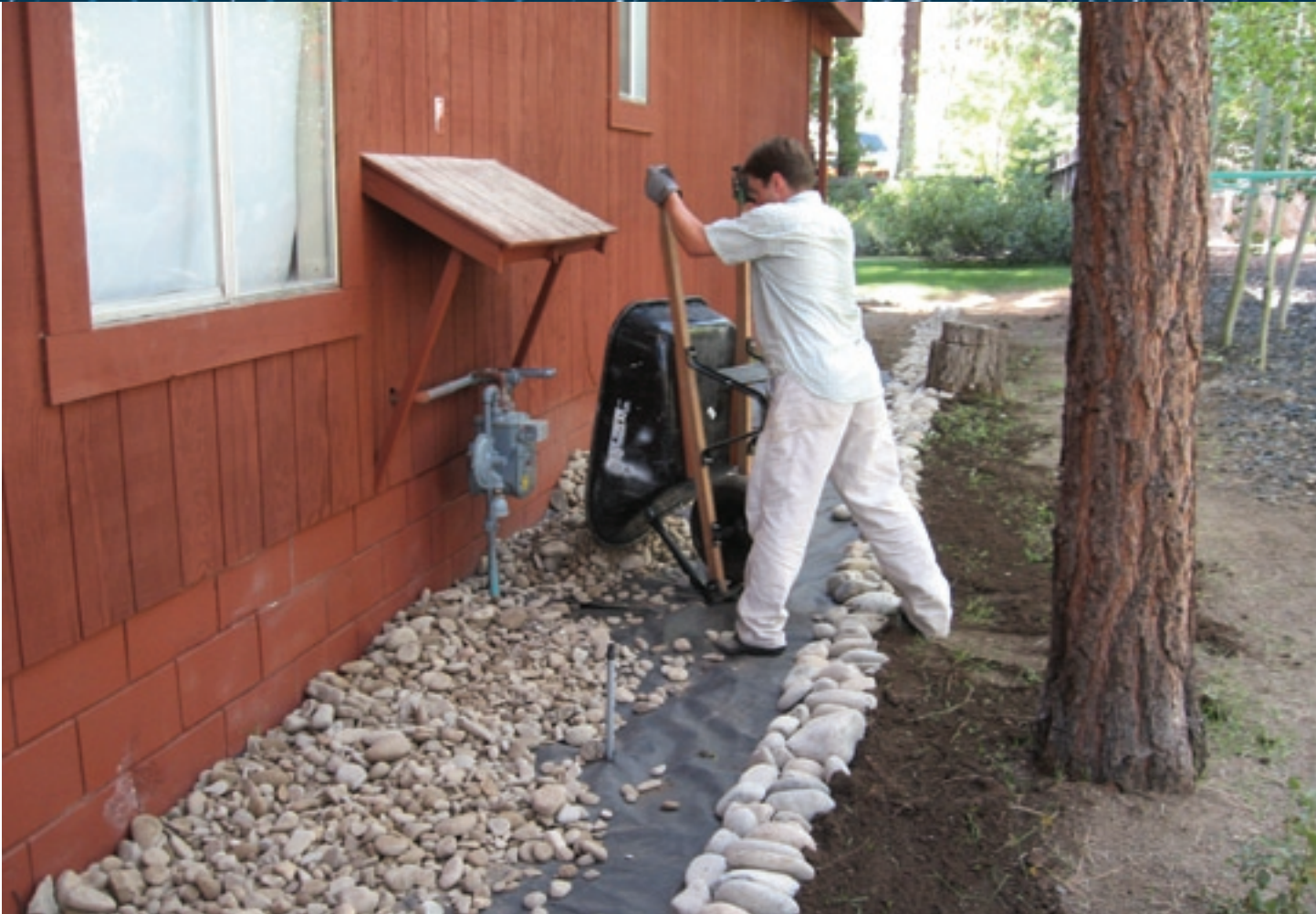
An armored drip line installed around a home in the Lake Tahoe Basin captures rainfall and keeps it on site, reducing runoff from the residential property.
