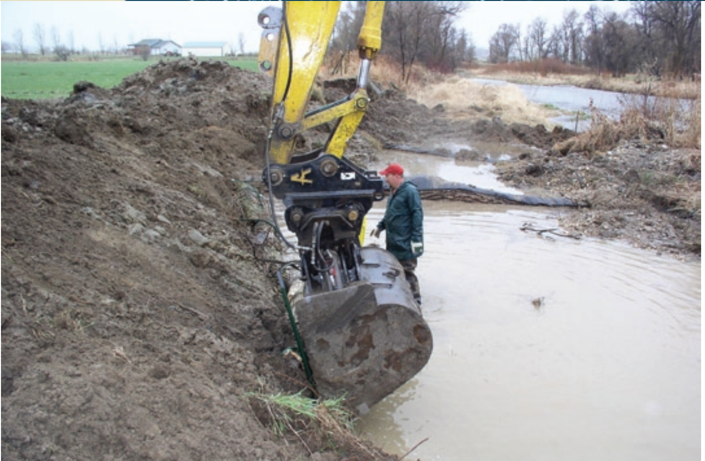
Streambank restoration work on the Tongue River is part of an effort to improve watershed health in Sheridan County, Wyoming.
