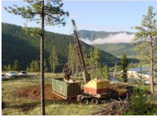
Figure 26—Crane loading loose landing slash pile material into large “dumpster-style” container. (Photo courtesy of Craig Rawlings, Montana Community Development Center.)
