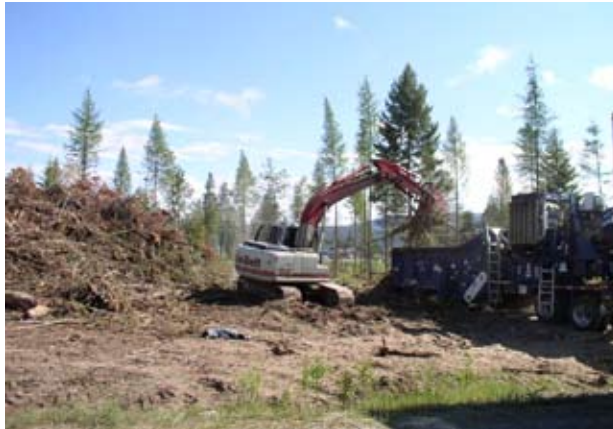
Figure 27—Small excavator used to load loose landing slash pile into a horizontal grinder. (Bonners Ferry, Idaho, 2006).
