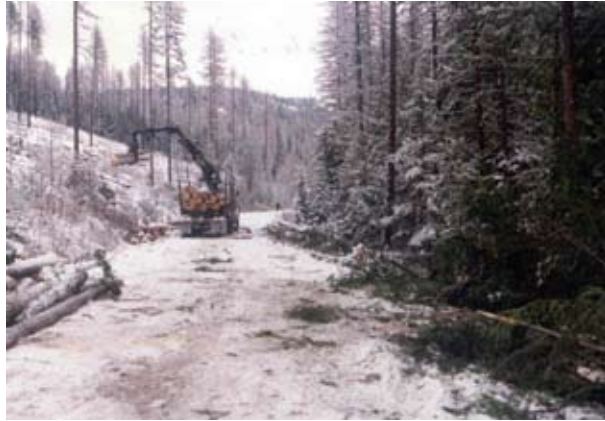
Figure 39—Solution, remove brush and trees using Section 31.12 (4) and a commercial timber sale contract to make room for snow removal. Treatment is taking place on the RIGHT side of the photo!
