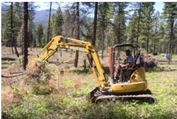
Figure 24—Mini-excavator normally used for piling slash could toss biomass in off-road-capable trailer.
