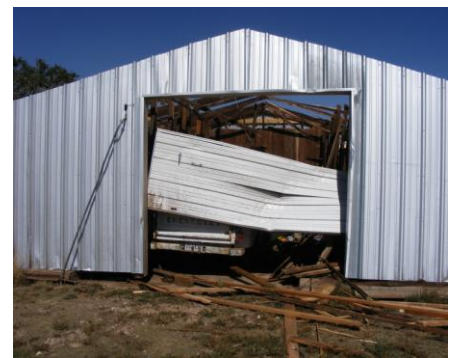
Fig. 1. Barn damaged by late season tornado
