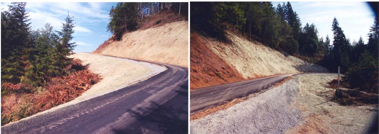
A portion of the ERFO repair on the Elk Mountain Loop Road.
