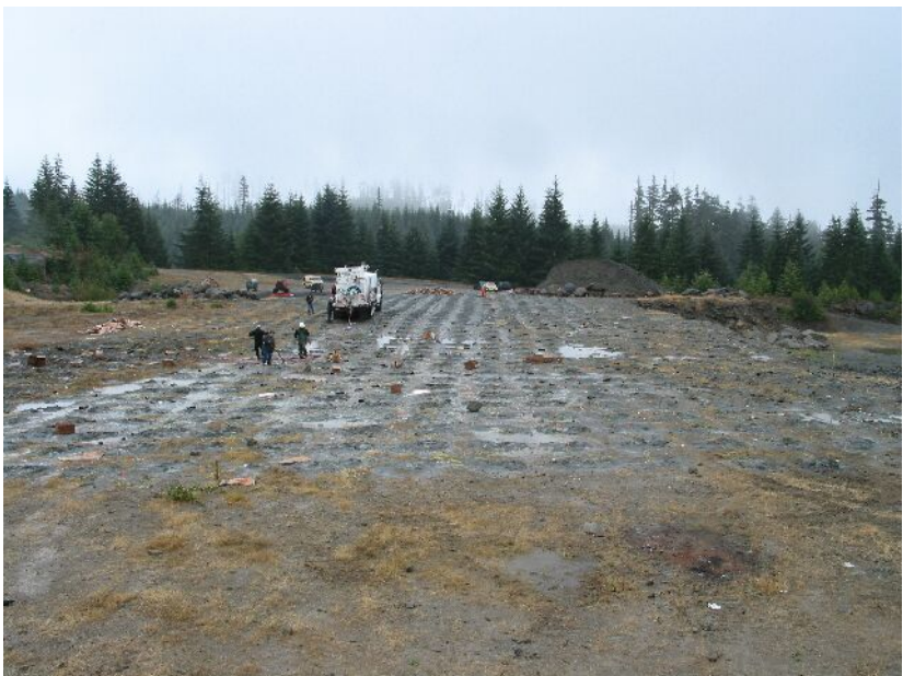
Packing drill holes with explosives at Elk Wallow Quarry before the 'shot'
