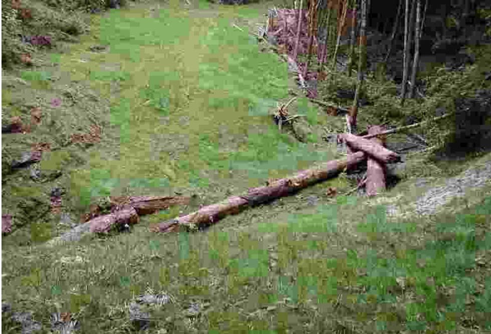
Figure 6. Wimer Creek road decommissioning. Culvert removed, slopes re-contoured, logs placed in stream, and soils stabilized.
